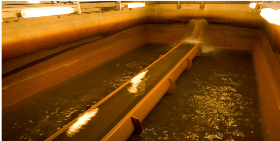
Figure 6.1: A Sand Filter in Operation in Denmark [42]
